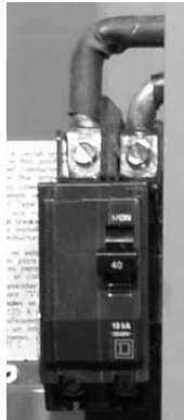
QO2100 Tenant Circuit Breaker Installed
