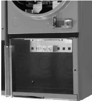
Branch Unit Load Equipment Grounding Terminals
