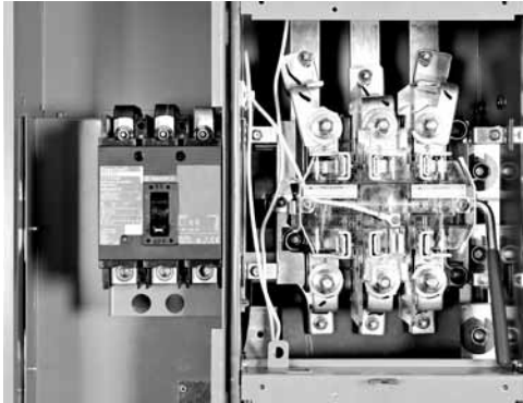
Q-Frame Circuit Breaker Installed
