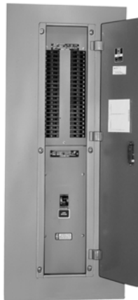
225 A Main Circuit Breaker
