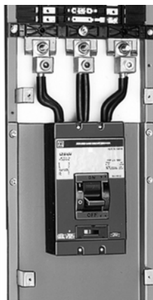
400 A Main Circuit Breaker Interior
