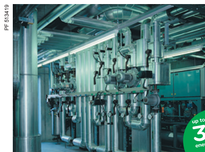
ATV12 controlling a pumping station
