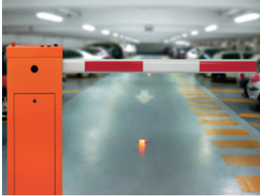
ATV12 controlling an access barrier
