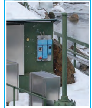
Hydroelectric power plant
