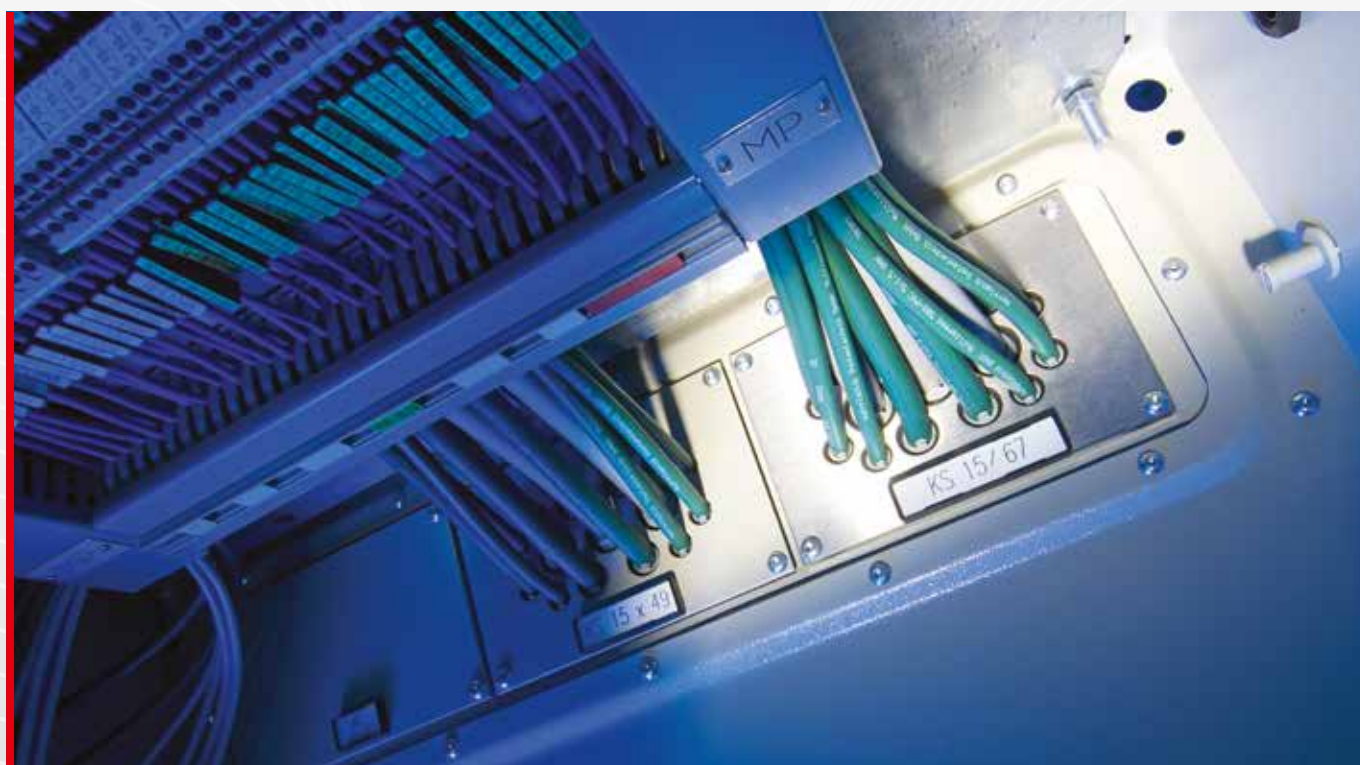
KDP 105/15 in the control cabinet
