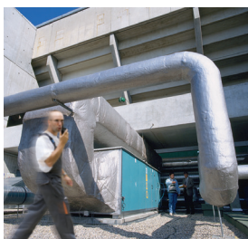
Air handling unit
